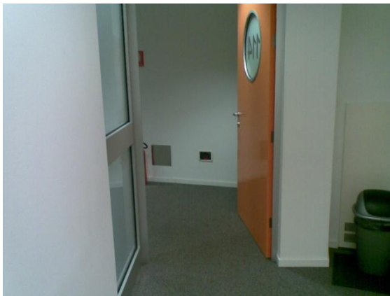
Figure 29 - The photograph shows an entrance door which is easy to open and clearly marked with large numbers.
