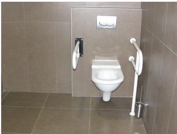
Figure 18 - The photograph shows an accessible toilet with grab bars and sufficient maneuvering space.
