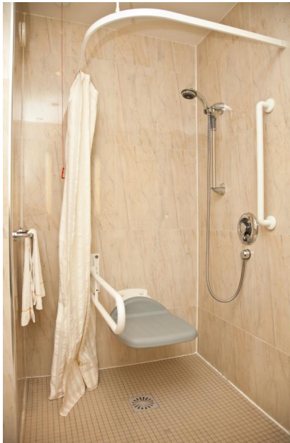
Figure 20 - The photograph shows an accessible shower area with a waterproof folding seat, a grab bar and an alarm ( http://jordanbuildersandjoiners.co.uk/disabled-access/ ).
