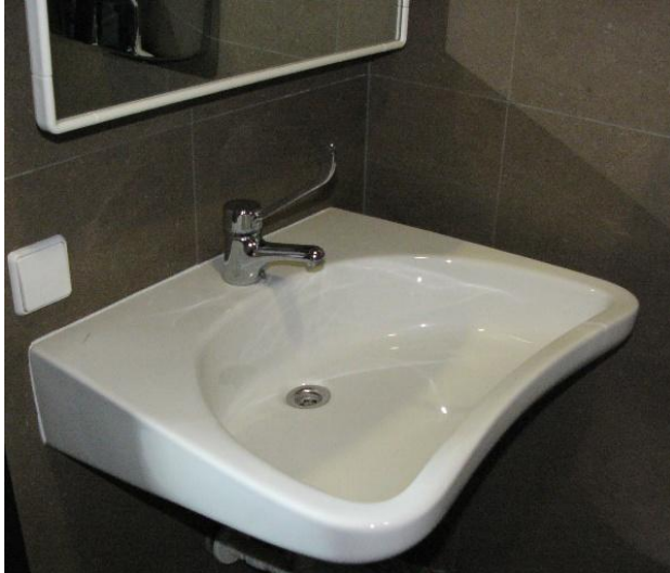
Figure 19 - The photograph shows an accessible washbasin with an ergonomically shaped single lever mixer tap.
